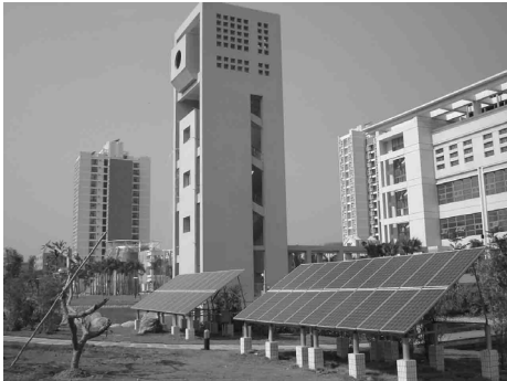
Fig. 4. Stand-alone solar pumping experimental systems in Shenzhen
