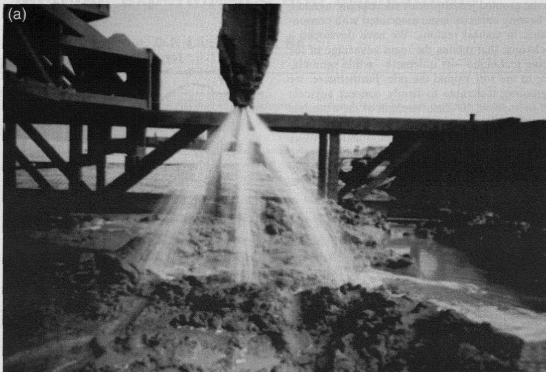
Fig. 2. New jetting methods for jetting of water from internal pipe within piles. (a) Jetting of water from one nozzle at a toe of a pile in the form of a cone. (b) Jetting of water from many smaller nozzles at a concrete sheet pile toe in the form of many downward flow lines with high speed.
