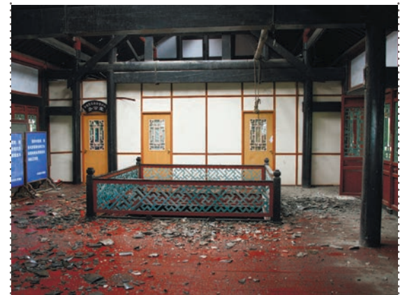
INTERIOR VIEW OF DAMAGE OF THE SECOND FLOOR BEFORE CONSERVATION
