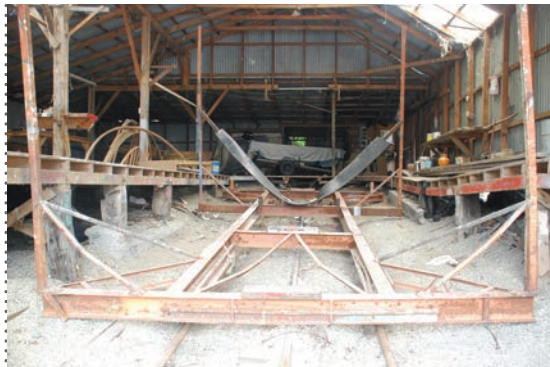
BEFORE: LARGER SLIPWAY LOOKING FROM THE LAKE. NOTE THE DISTORTION IN THE TIMBER FLOOR ON THE RIGHTHAND SIDE.
