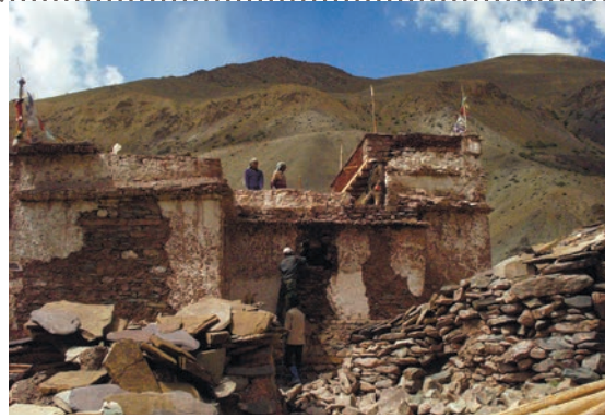
STITCHING CRACKS AND REPAIRING DILAPIDATED MASONRY OF THE TEMPLE WALLS AND PARAPET
