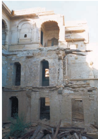
EXTERNAL WALL BEFORE CONSERVATION
