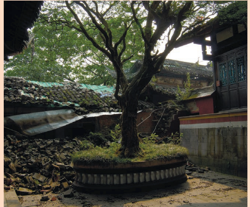
STRUCTURAL DAMAGE AFTER EARTHQUAKE
