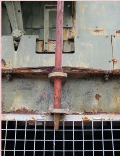
METAL ELEMENTS AFFECTED BY SALTWATER CORROSION
