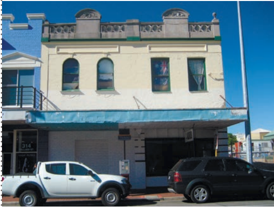
KURB GALLERY BEFORE CONSERVATION
