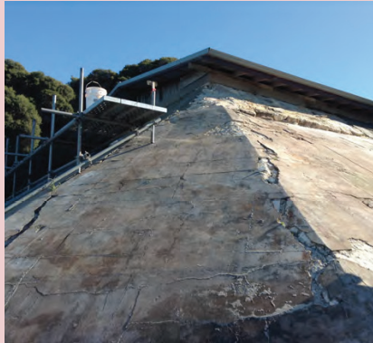
CONCRETE DETERIORATION AT F1 MAGAZINE
