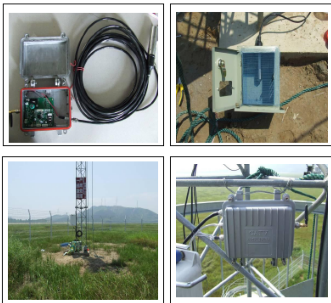
Figure 9. The installation pictures of the RWMS at Poyanghu Lake.
