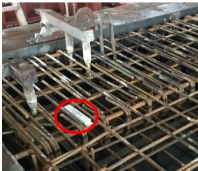
(g) RFID installation
