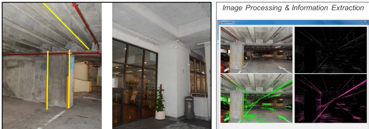
Figure 5 Structural components in a typical building (photos taken by author in 2016) (left part); Image processing and information extraction using Hough Transformation (right part)
