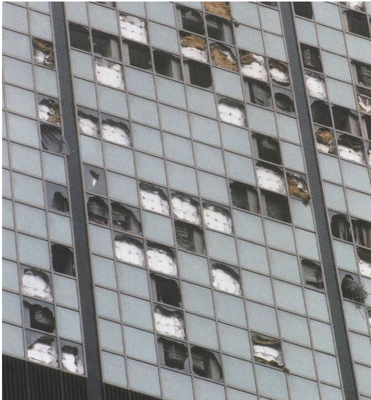
Figure 4. Window damages during Typhoon York 1999
