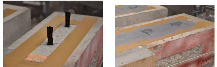
(a) Installation of anchors (b) Installation of FRP plate Figure 4. Construction of test specimens.
