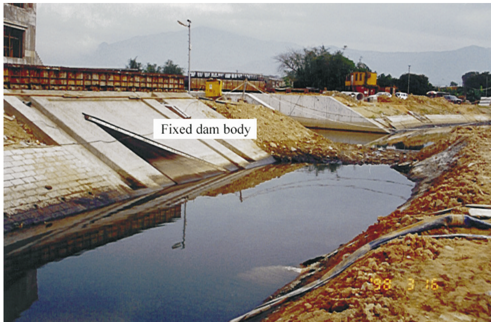
Fig. 1. Water flowing over fixed rubber dam body.
